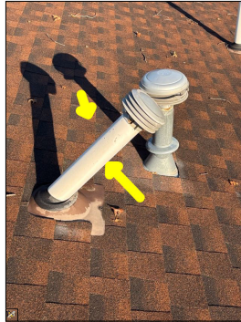
Flue is unconventionally crooked and not plumb. This is considered abnormal and amateur craftsmanship. Amateur craftsmanship is prone to failure.
