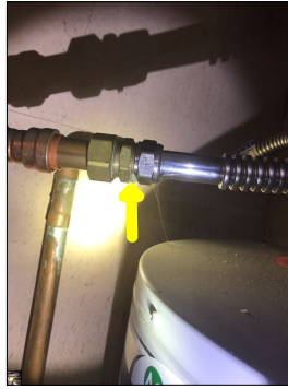
Corrosion along the water supply lines.
