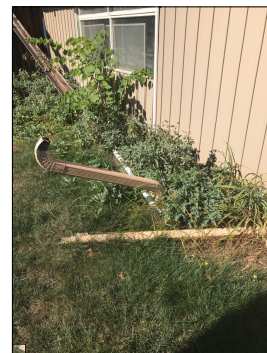
Damaged gutter system.
