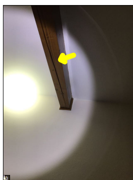
Split along the beam.
