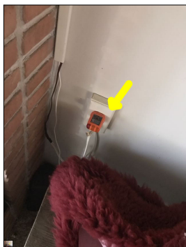
The receptacle is inoperable.
