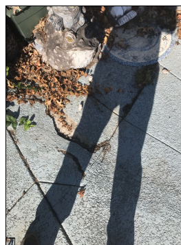
Cracks and deterioration along the service walks.
