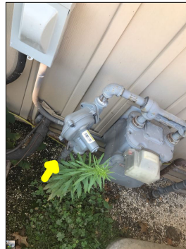
Main fuel shut off valve.
