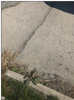
Cracks and deterioration along the driveway.
