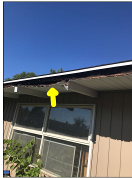
Gaps along the siding.
