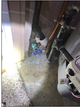
Apparent main water shut-off valve.
