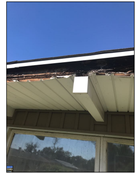
Wood rot damage.
