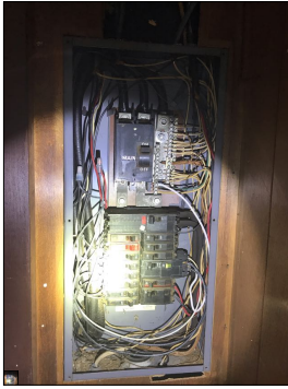
General photo of the panel in the detached garage.
