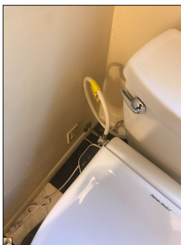
Non GFCI protected receptacles.
