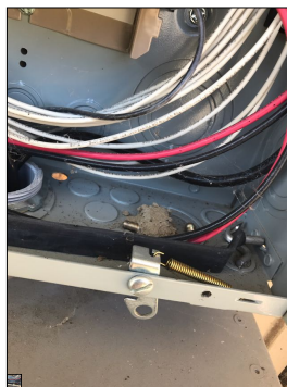
Apparent wasp nest within the electrical panel. Wildlife activity can cause property damage.
