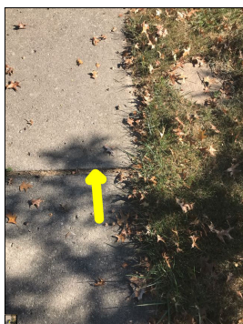
Uneven surfaces along the service walks.
