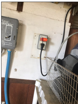
Non GFCI protected receptacles.
