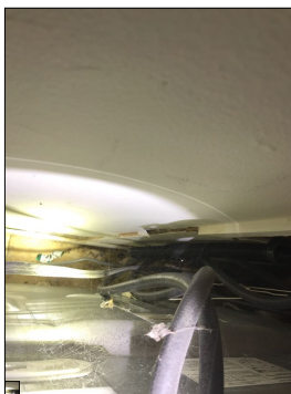
Damage observed along the wall behind the washer.
