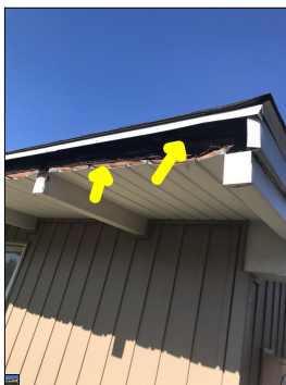
Wood rot damage along the sheathing. An active or intermittent water source can cause mold growth, wood rot, and property damage.
