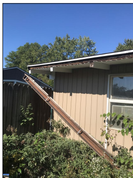
Damaged gutter system.
