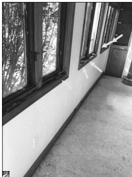
Missing window cranks, thus making the windows inoperable.
