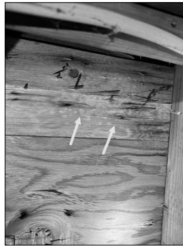
Mold like substance along the sheathing/framing. An active or intermittent water source can cause mold growth and property damage, such as wood rot damage.
