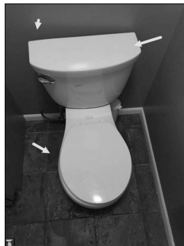
The toilet is crooked. This is considered abnormal and amateur craftsmanship.
