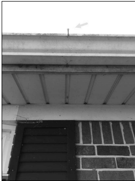
Loose gutter spikes.
