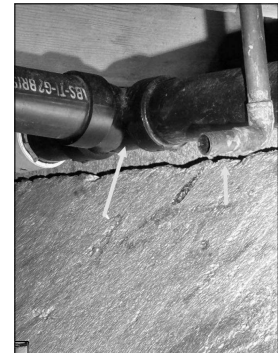
Improper horizontal plumbing transition. This is considered amateur craftsmanship. A sanitary wye should be used for horizontal plumbing transitions. The use of improper plumbing transitions can create slow drainage and potential blockage. Also, there is an open ended plumbing pipe. This is considered abnormal.
