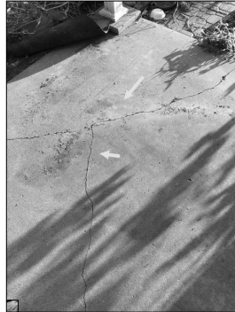
Cracks and deterioration along the patio.
