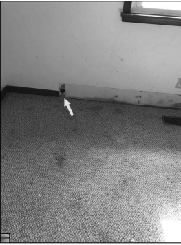
Holes/damage along the wall.
