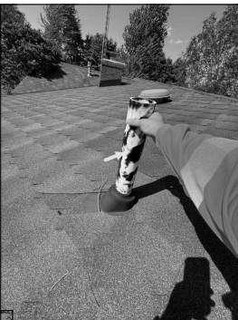
The plumbing vent is loose. It can move back and forth. Plumbing vents should not have any movement and be fully secured.
