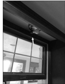
The light is inoperable.
