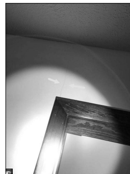
Cracks along the walls.
