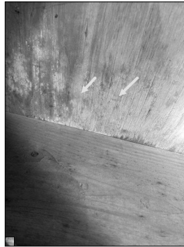
Mold like substance along the subfloor. An active or intermittent water source can cause mold growth and property damage.
