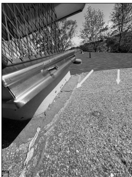
Cracks along the chimney. Cracks are considered defects and potential leak points.
