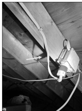
Electrical extension cords observed in the attic. Extension cords in the attic is considered a safety/fire hazard. Extension cords should not be used as permanent wiring.
