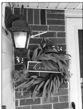
The light flickers. This is considered a defect.
