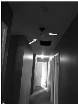
The light is inoperable.
