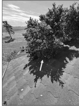
Vegetation in proximity of the roof. Falling branches can damage the roof system. Also, vegetation in proximity of the roof can enable small animals and rodents access to the roof. Wildlife activity can cause property damage.
