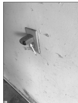
Non GFCI protected receptacles.
