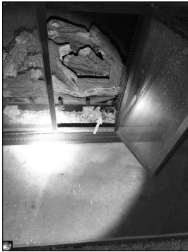
The fireplace is a gas fireplace. There is no apparent electronic ignition. It is beyond the scope of a general home inspection to light fuel burning appliances. Doing so could cause property damage. Recommend a licensed chimney/fireplace professional further evaluate to make sure the fireplace is in good working condition and safe to use.
