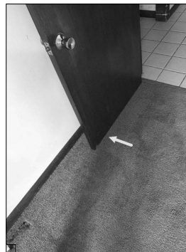
The door drags the floor during operation.
