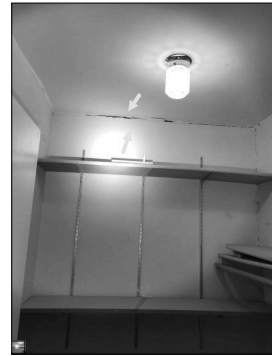
Damage along the ceiling.
