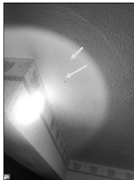
Discoloration along the ceiling.
