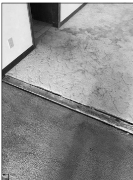
Uneven surfaces along the floor. Uneven surfaces are a potential trip hazard.
