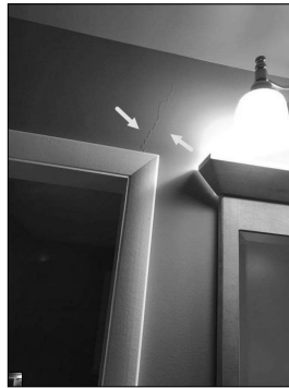
Cracks along the walls.
