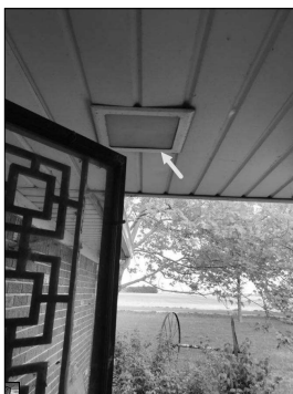
The light is inoperable.
