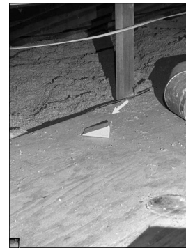
Pest control. Wildlife activity can cause property damage.
