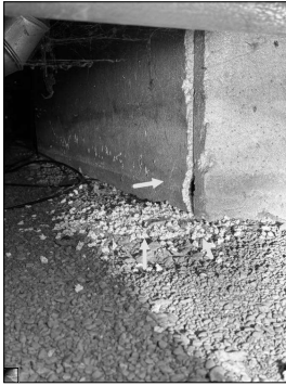
Damaged insulation. This is a sign of wildlife activity.
