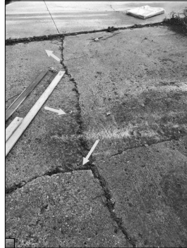
Cracks and deterioration along the driveway.
