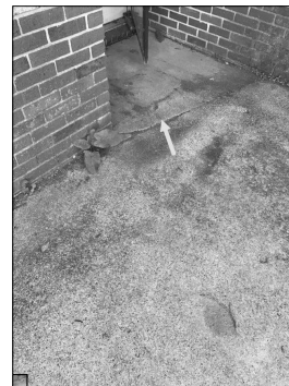
Cracks and deterioration along the porch.
