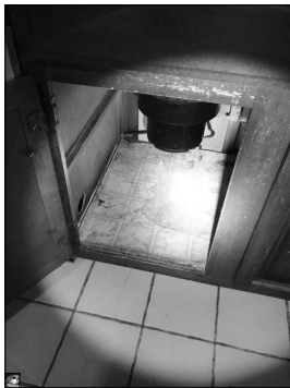
The garbage disposal is inoperable.
