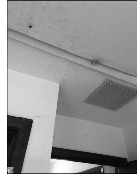
Cracks along the ceiling.
