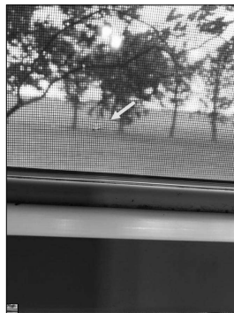
Holes along the window screen.
