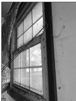
Excessive debris along the windows.
