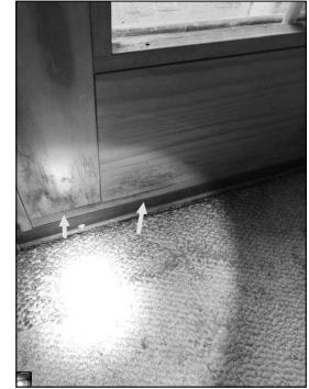
Mold like substance along the door. An active or intermittent water source can cause mold growth and property damage.
