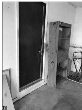
The door that separates the interior of the house from the garage is not a proper fire rated door. This is a potential safety hazard.
