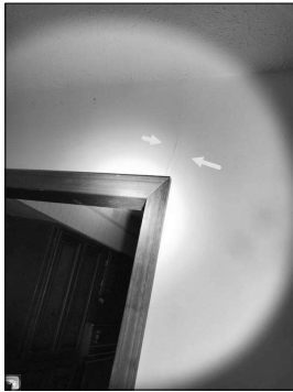
Cracks along the walls.
