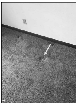
The floor is spongy and moves when walking on it. This is considered abnormal and a defect.
