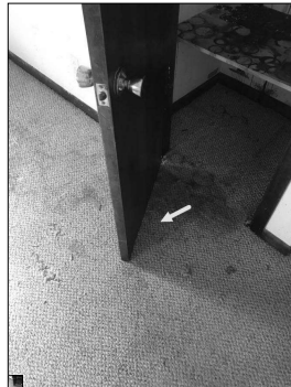
The door drags the floor during operation.
