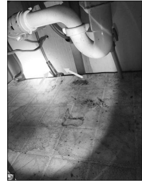
The spray hose is unconventionally located under the sink.
