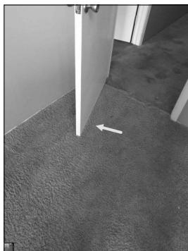
The door drags the floor during operation.
