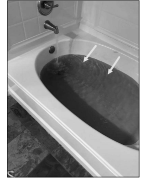
The water is unconventionally dark. This is considered abnormal and a defect.
