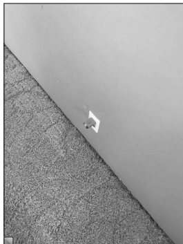
Open ground receptacles.
