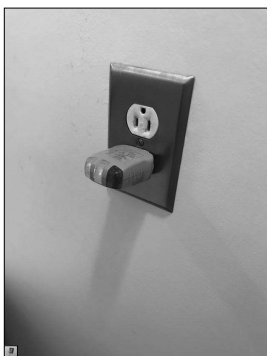
Non GFCI protected receptacles.
