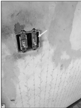
Missing switch covers.
