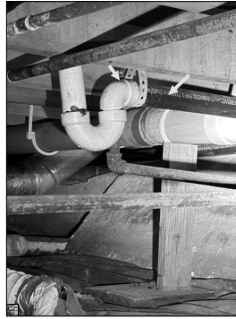
Two different types of plumbing materials joined together. This installation has ABS and PVC connected together. When difficult types of plumbing materials are glued together, they are prone to creating a poor seal, thus creating leaks.
