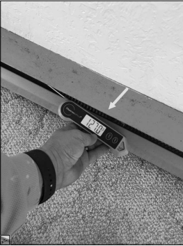
The electric baseboard is operable.
