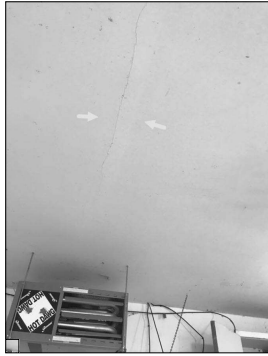
Cracks along the ceiling.
