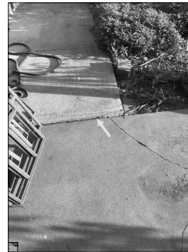
Uneven surfaces along the service walks.
