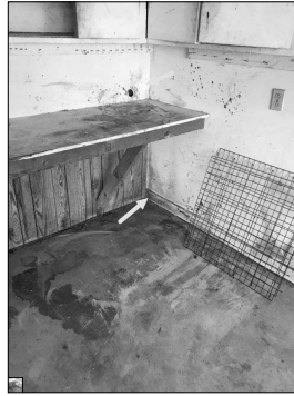
Discoloration along the walls. Also, hole along the wall.
