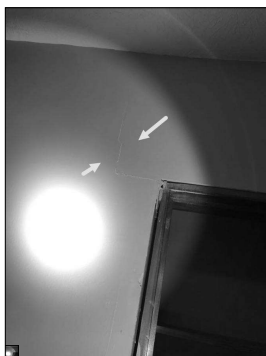
Cracks along the walls.
