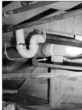
The plumbing pipe is unconventionally supported by a board wedged underneath the pipe. This is considered abnormal and amateur craftsmanship.
