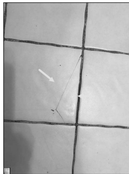
Cracked floor tiles.
