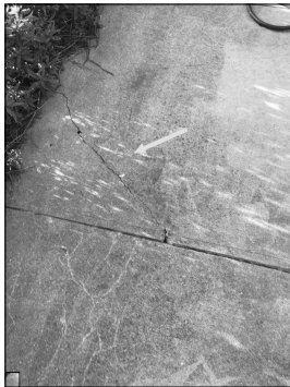
Cracks and deterioration along the service walks.
