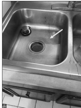
Slow sink drainage. This is considered a defect.
