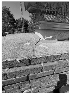
Deterioration and cracking along the brick. Also, deterioration and cracking along the clay tile. Cracks and deterioration along the clay tile can cause improper drafting, thus creating a safety hazard.
