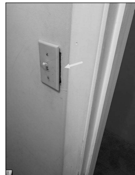
The switch cover is not flush with the wall. This is considered a defect and a potential safety hazard.
