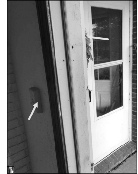
The wall switch does not turn off the adjacent exterior light. Nor does the wall switch in the laundry room either. This is considered abnormal and a defect.
