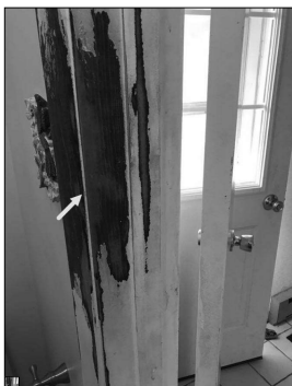
Discoloration along the door.
