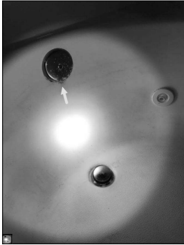
Discoloration along the bathtub.
