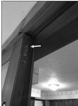
The door does not latch properly.
