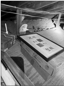
Debris and clutter within the attic. Visibility and accessibility were limited.
