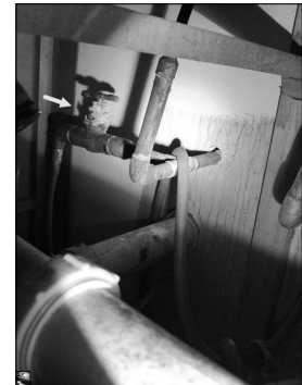
Rust/corrosion along the plumbing pipes.
