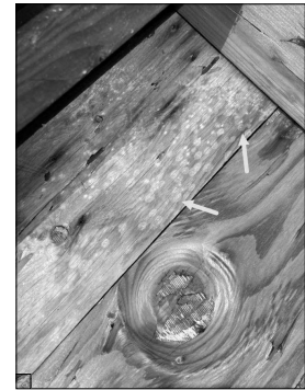
Mold like substance along the sheathing/framing. An active or intermittent water source can cause mold growth and property damage, such as wood rot damage.
