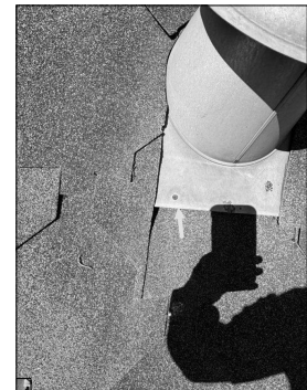
Exposed nailheads/staples. Exposed nailheads/staples are potential leak points.
