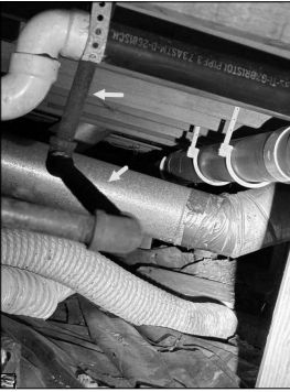
Rust and corrosion along the fuel lines. Rust and corrosion can create holes along the fuel lines, thus creating fuel leak.
