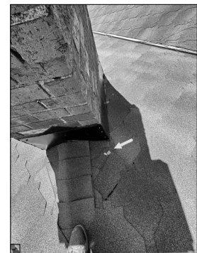
Deterioration and cracking along the chimney. Deterioration and cracks are potential leak points.
