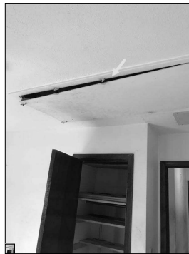
The attic access stairs sag. This is considered a defect.
