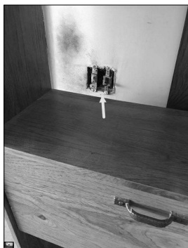
Missing switch cover.
