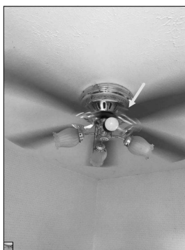
The ceiling fan is operable, however, the light is inoperable.
