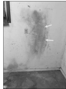
Discoloration along the wall. Discoloration along the ceiling is considered abnormal and a defect. An active or intermittent water source can cause discoloration, mold growth and property damage.
