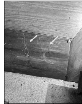
Mold like substance along the band joist. An active or intermittent water source can cause mold growth and property damage.
