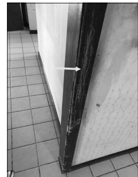
Scratch marks along the walls.
