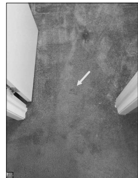
The floor slopes. This is considered abnormal and a defect.
