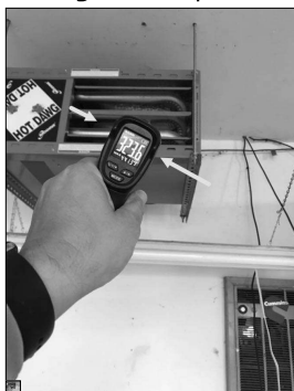
The garage heater is operable.
