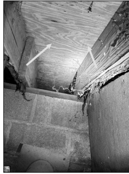
There is no insulation along the subfloor. This is not a recommend practice. The lack of insulation does not meet the industry standard. An insulated subfloor can help maintain desired room temperatures within the above living areas, thus reducing utility expenses with heating and cooling.
