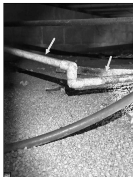
Negative slopes along the condensation drain pipe. This is not a recommended practice and does not meet the industry standard. A negative sloped drain pipe can cause slow drainage and possible blockage.
