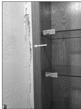
Flaking and peeling along the walls.
