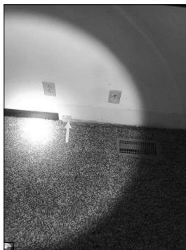
Damage along the wall.
