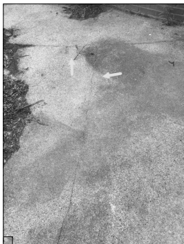
Cracks and deterioration along the porch.
