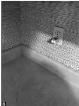
Non GFCI protected receptacles.
