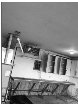
The light is inoperable.
