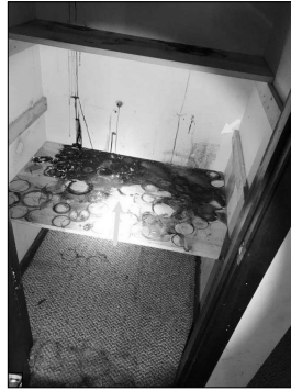
Discoloration along the wall. Discoloration along the wall is considered abnormal and a defect. An active or intermittent water source can cause discoloration, mold growth and property damage.
