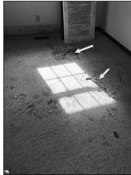
Torn floor covering.
