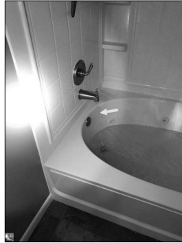
The bathtub faucet leaks while the showerhead is in operation. This is considered a defect. A properly functioning diverter will not allow any water through the bathtub faucet while the showerhead is in operation.
