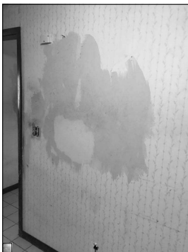
Discoloration along the walls.
