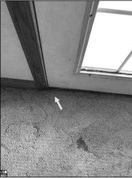
Torn weatherstrip along the door.
