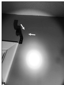
Cracks along the walls.
