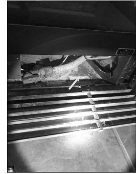
Mice droppings observed underneath the fireplace. Wildlife activity can cause property damage.
