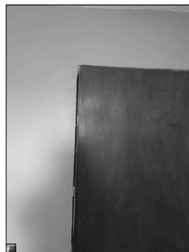
The door does not properly close.
