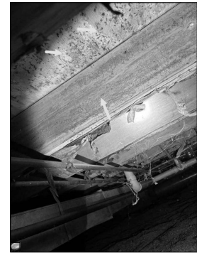
Mold like substance along the floor joists. An active or intermittent water source can cause mold growth and property damage.
