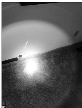
Holes/damage along the wall.
