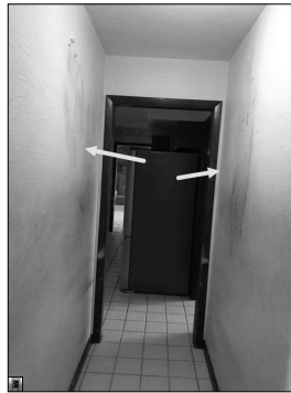
Discoloration along the walls.
