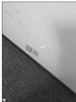
The receptacle is not flush with the wall.
