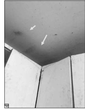
Discoloration along the ceiling. Discoloration along the ceiling is considered abnormal and a defect. An active or intermittent water source can cause discoloration, mold growth and property damage.
