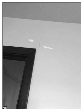
Cracks along the walls.
