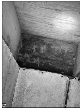
Mold like substance along the band joist. An active or intermittent water source can cause mold growth and property damage.
