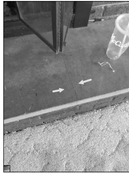
Crack along the hearth.
