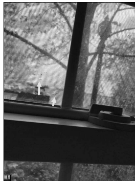
Holes along the window screens.
