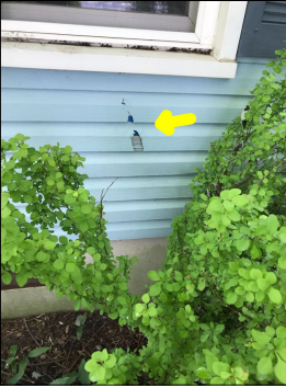
Holes along the siding.
