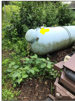
Main fuel shut off valve.
