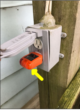
Open ground receptacle.
