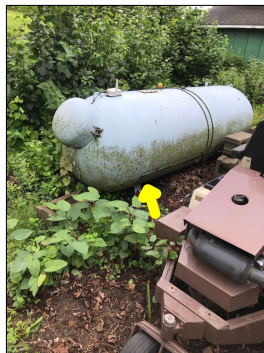
The fuel tank has rust and corrosion along it. The fuel tank is considered aged.
