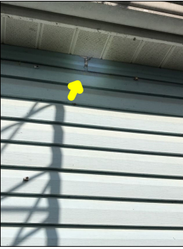
Gaps along the siding.
