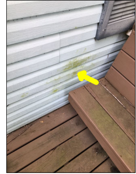
Discoloration along the siding.
