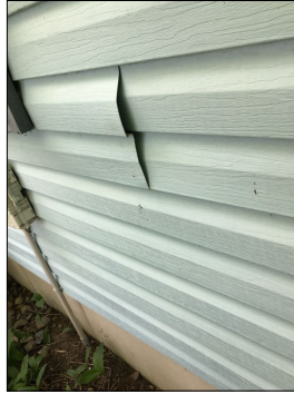
Gaps along the siding.
