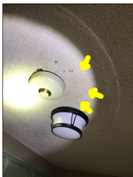
Discoloration along the ceiling.
