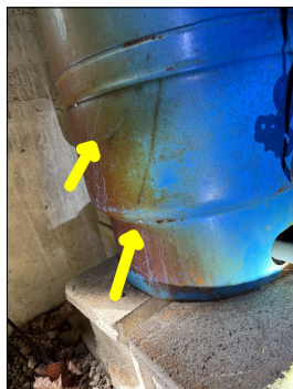
Rust/corrosion along the pressure tank.
