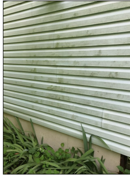
Discoloration along the siding.
