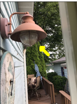
The light is inoperable.
