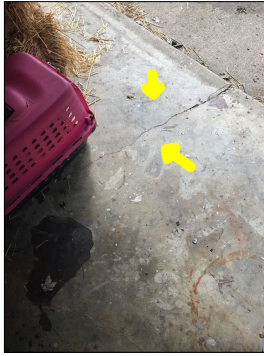
Cracks and deterioration along the floor.
