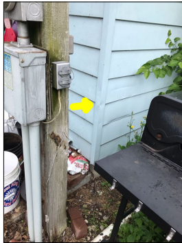
Dents along the siding.
