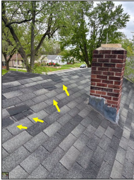
Loose/detached roof shingles.
