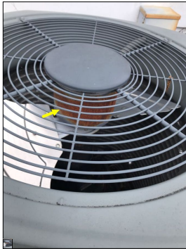
Rust and corrosion along the condenser.
