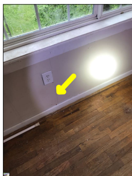
Cracks along the walls.
