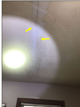
Cracks along the ceiling.
