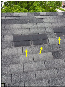
Loose/detached roof shingles.
