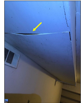
The ceiling is sagging.
