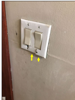
Cracked and damaged cover.
