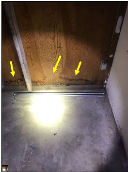
Discoloration along the wall and signs of previous water damage. An active or intermittent water source can cause mold growth and property damage.
