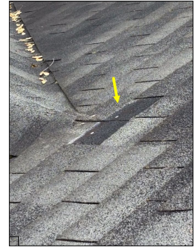
Missing roof shingles. Missing shingles can allow water intrusion into the house. An active or intermittent water source can cause mold growth and/or property damage.
