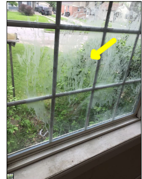
Discoloration along the window.
