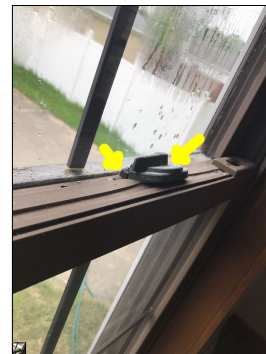
The window lock is unconventionally bent.
