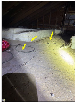
Electrical extension cords observed in the attic. Extension cords in the attic is considered a safety/fire hazard. Extension cords should not be used as permanent wiring.
