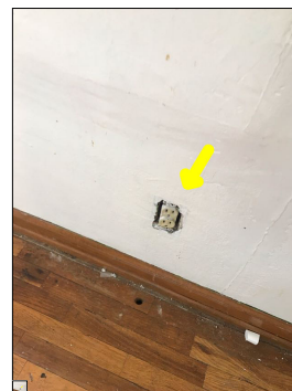
Missing receptacle cover.
