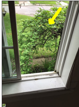
Missing window screens.
