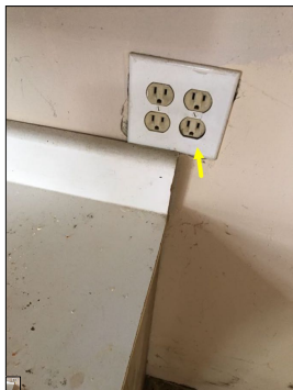
Recessed receptacles. Recessed receptacles are considered amateur craftsmanship and a defect.
