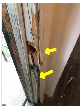
Damaged door frame.
