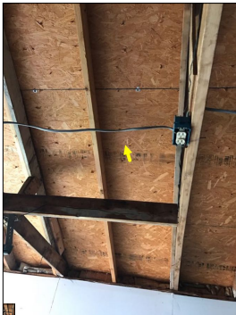
The wires are not wrapped in conduit. This is considered abnormal, amateur craftsmanship and a potential safety hazard. Wires should be wrapped in conduit to protect both humans and the electrical wiring. Wires that lack conduit can potentially get pulled, become loose, or damaged, thus creating shock hazards and/or fire hazards.
