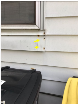
Exposed nails/fasteners along the siding. Exposed nails/fasteners are potential leak points. Exposed nails along the siding is considered amateur craftsmanship. Amateur craftsmanship is prone to failure and leakage.
