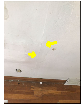
Cracks along the walls.
