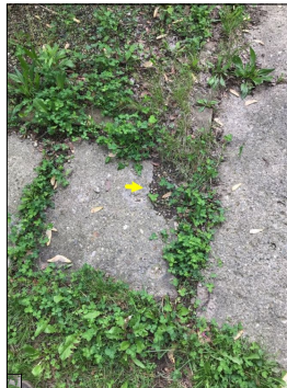
Cracks and deterioration along the service walks.
