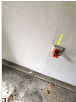
Non GFCI protected receptacles.
