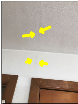
Cracks along the ceiling and walls.
