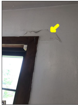
Flaking and peeling along the walls.
