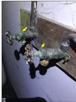
Rust/corrosion along the washer hook up lines.
