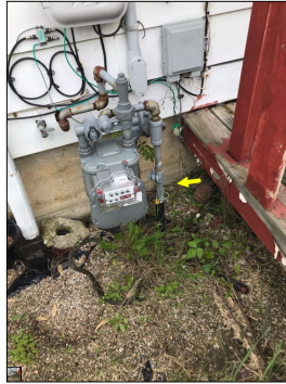
Main fuel shut off valve.
