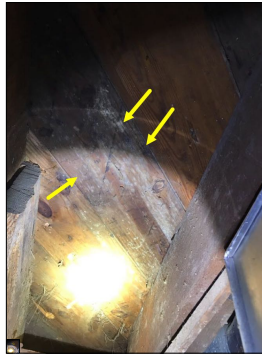
Mold like substance along the subfloor. An active or intermittent water source can cause mold growth and property damage.
