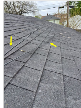
Cables resting along the roof. This is considered abnormal and does not meet the industry standard.
