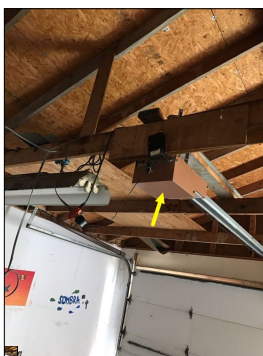
The automatic opener is inoperable.
