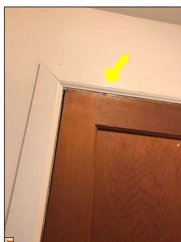
The door sticks and is difficult to operate.
