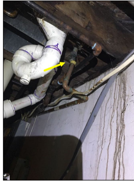
Ruptured water supply line.
