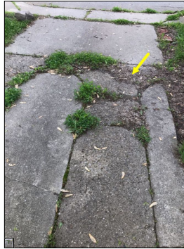
Cracks and deterioration along the driveway.
