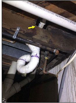
Unconventional notches and alterations along the floor joists. This is not a recommended practice. The unconventional notches and alterations can compromise the structural integrity of the floor joists, thus resulting in squeaky floors, sloped floors, cracks along walls and ceilings, doors and windows not properly closing and opening, etc.
