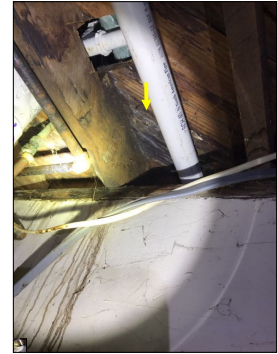
Discoloration along the floor joists/subfloor. Discoloration can be a potential mold like substance. An active or intermittent water source can cause discoloration, property damage and mold growth.
