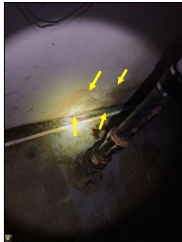
Mold like substance. An active or intermittent water source can cause mold growth and property damage.
