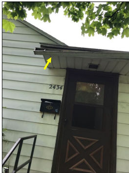
Dents/damage along the gutter system.
