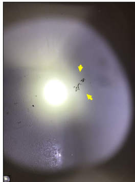
Chips/damage along the bathtub. Chips and damage are considered defects and are potential leak points.
