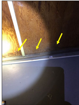
Discoloration along the wall. Discoloration along the wall is considered abnormal and a defect. An active or intermittent water source can cause discoloration, mold growth and property damage.
