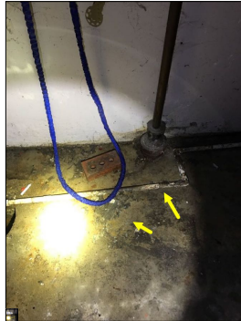
Moisture/dampness observed. This is considered a defect. An active or intermittent water source can cause mold growth and property damage.
