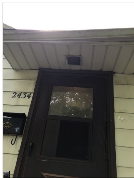
The light is inoperable.
