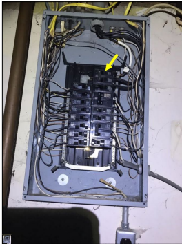
Main circuit breaker.
