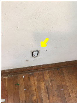
Missing switch cover.
