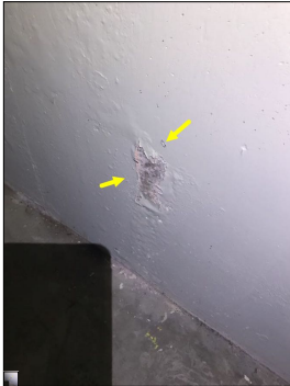
The wall is flaking/bubbling. This is considered abnormal and a defect. An active or intermittent water source can cause flaking and bubbling.
