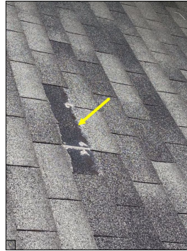
Missing roof shingles. Missing shingles can allow water intrusion into the house. An active or intermittent water source can cause mold growth and/or property damage.
