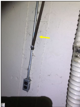
The fuel line does not have a shut off valve adjacent to where the dryer would be located. This is a potential safety hazard.
