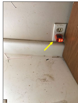
Non GFCI protected receptacles.
