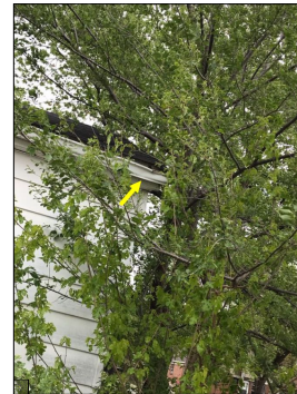
Dents/damage along the gutter system.
