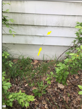
Dents along the siding.
