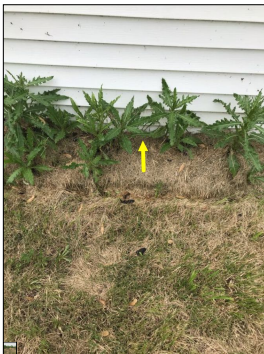
The siding is in proximity to the ground. Siding should have at least 6 to 8 inches of clearance above the ground. Maintaining proper clearances reduces access to wood structures behind the siding and helps preserve the house. The proper clearances help restrict access from wood destroying insects and/or moisture/water that might find its way behind the siding.
