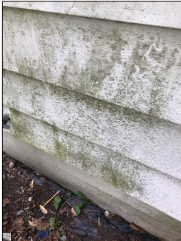
Discoloration along the siding.
