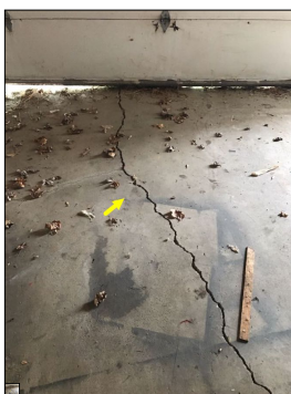
Cracks and deterioration along the floor.
