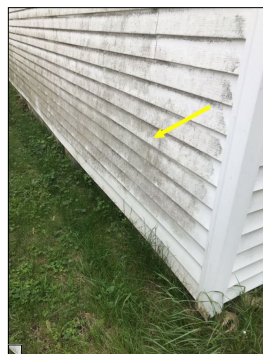
Discoloration along the siding.
