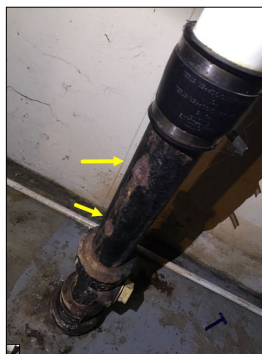
Rust and corrosion along the plumbing pipes.
