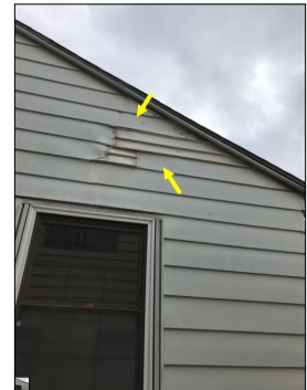
Unconventional repairs along the siding.
