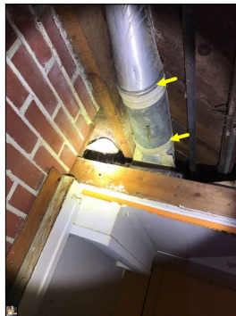
Potential asbestos based tape along the ductwork. Asbestos is a potential safety hazard.
