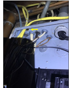
Wires routed through the knockout without a bushing or clamp. This is considered a safety hazard as the metal edge of the knockout could penetrate the wires, thus causing spark and a fire.
