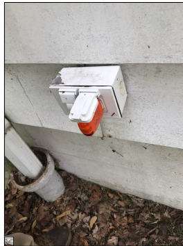
Non GFCI protected receptacles.
