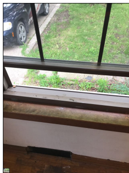
Missing window screens.
