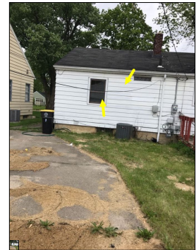
The cables are unconventionally low.
