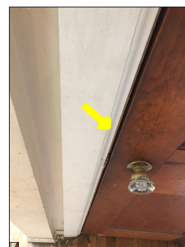
The door does not latch properly.
