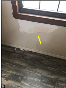
Flaking and peeling along the walls.
