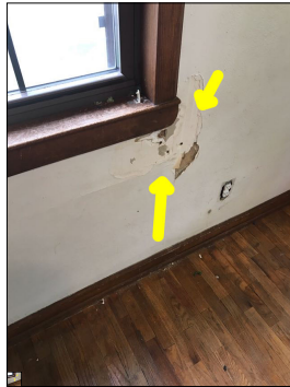
Damage along the wall.
