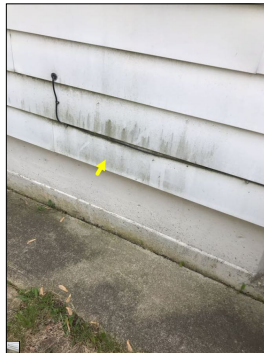
Discoloration along the siding.
