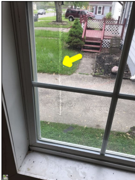
Holes along the window screen.
