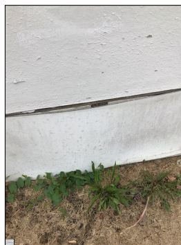
Deterioration along the overhead door.
