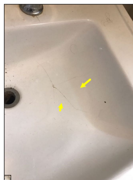
Cracks along the sink.
