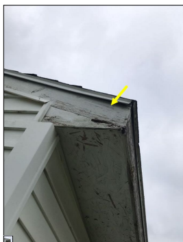
Holes and deterioration along the siding.
