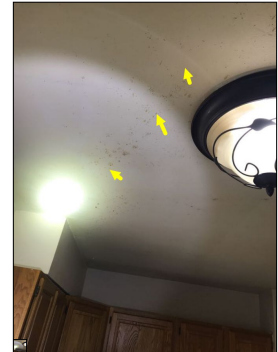
Mold like substance. An active or intermittent water source can cause mold growth and property damage.
