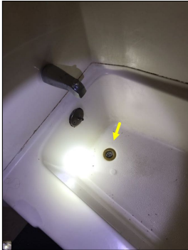
The drain is missing a grate/screen. The lack of a grate/screen over the drain can allow debris down the drain, thus potentially creating slow drainage or blockage.
