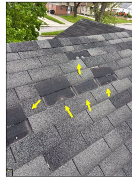
Loose/detached roof shingles.
