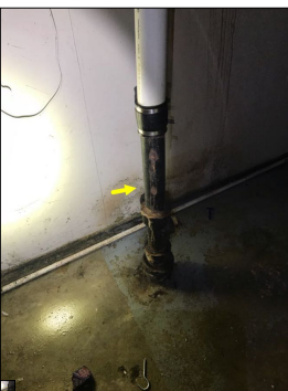
Aged cast iron drain pipes. Cast iron drain pipes no longer meet modern day plumbing standards. Cast iron pipes are prone to corroding from the inside out. Cast iron drain pipes are towards the end of their life expectancy. Repairs or replacement to cast iron drain pipes should be anticipated.
