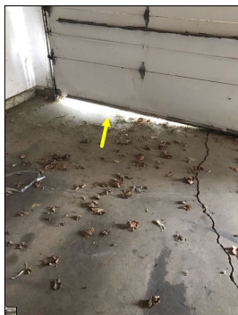
Daylight can be seen from the interior. This is an entry point for moisture, insects, mice, rodents, etc.
