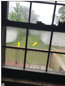
Insulated glass seal failure.
