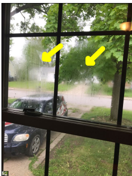
Insulated glass seal failure.
