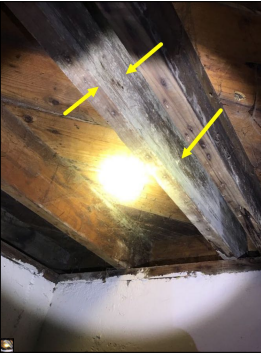
Mold like substance along the floor joists. An active or intermittent water source can cause mold growth and property damage.
