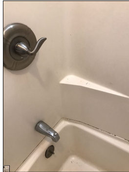
The showerhead and faucet are inoperable.
