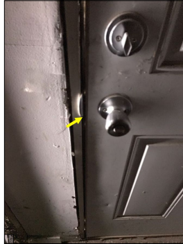
The door does not latch properly.
