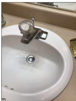
Inoperable drain stopper.
