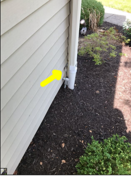
Detached downspout bracket.
