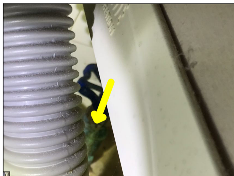
Rust/corrosion along the washer hook up lines.
