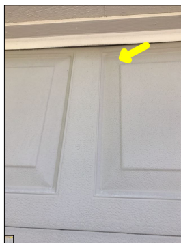
Dents/damage along the overhead garage door.
