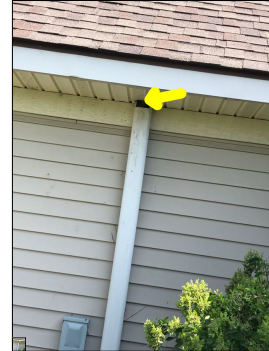
Gaps along the siding.
