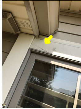
Cracks along the siding.
