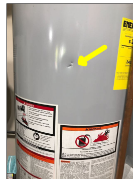
Dents along the water heater.
