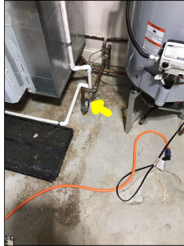
Main water shut off valve.
