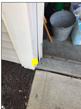
Gaps along the siding.
