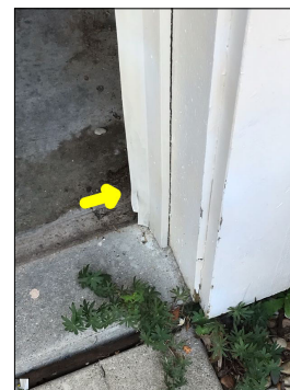
The weatherstrip is partially torn/missing along the overhead garage door. The lack of a proper weatherstrip can allow the intrusion of moisture, insects, wood destroying insects, mice and rodents into the property.
