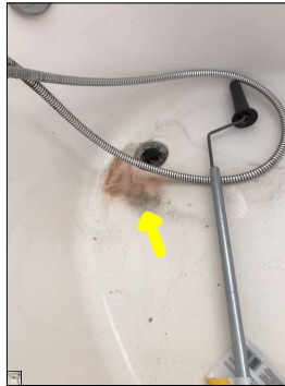
Discoloration along the bathtub.
