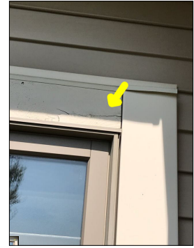
Cracks along the siding.
