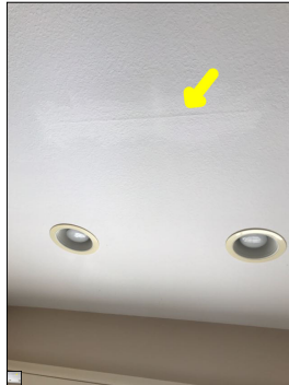
Cracks along the ceiling.
