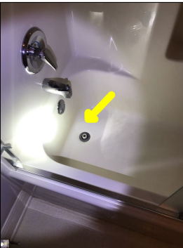
Inoperable drain stopper.
