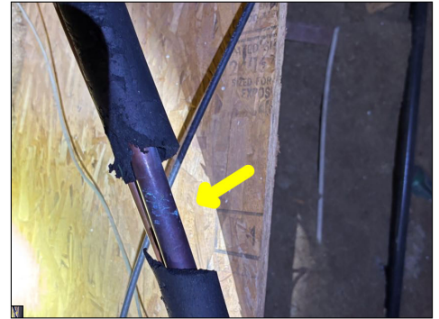
The insulation to the suction line is torn/missing. The insulation on the suction line is important so the refrigerant in the line does not absorb additional heat. The hotter the refrigerant, the harder the condenser has to work, thus shortening the life of the condenser. Also, the lack of insulation can allow the suction line to condensate at times. This can cause the suction line to have moisture drip from it. An active or intermittent water source can cause mold growth and property damage.
