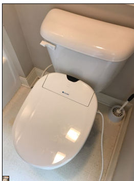
The toilet continuously calls for water. This is considered abnormal and a defect.
