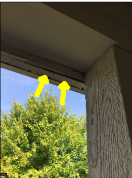
Wood rot damage.
