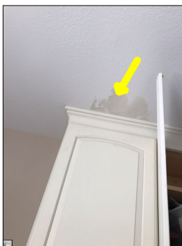
Discoloration along the ceiling.
