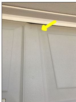
Dents/damage along the overhead garage door.
