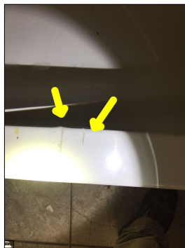
Damage along the bathtub.
