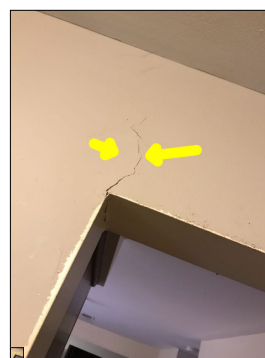
Cracks along the walls.
