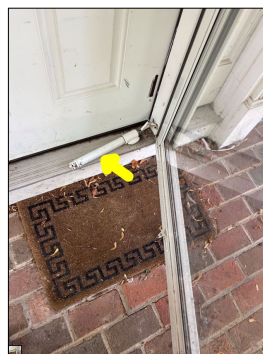
The suspension to the storm door is detached.
