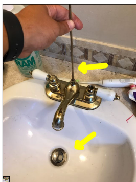
Inoperable drain stopper.
