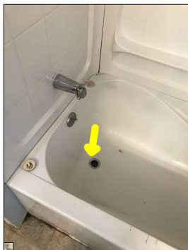
Missing drain stopper.
