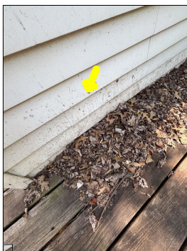
Discoloration along the siding.
