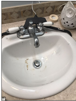
Inoperable drain stopper.
