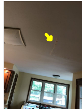
Cracks along the ceiling.
