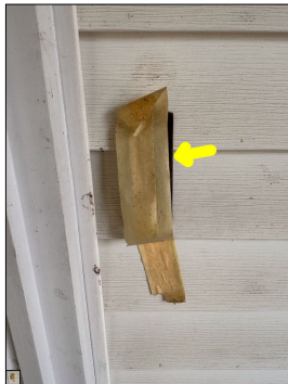
Unconventional tape along the door bell.
