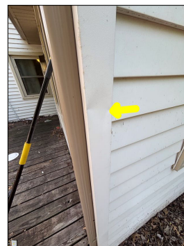
Dents along the siding.
