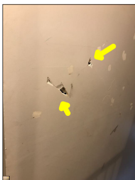
Holes along the walls.
