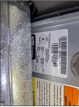
Furnace data plate.
