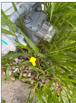
Main fuel shut off valve.
