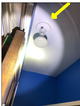
The light is inoperable.
