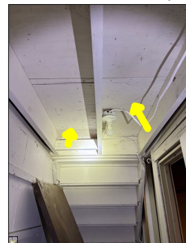
Some of the floor joists and subfloor have been painted/coated white. This could potentially be a form of previous mold remediation.
