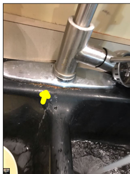
Rust/corrosion along the faucet/sink.
