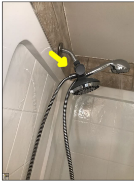
The showerhead leaks during operation.
