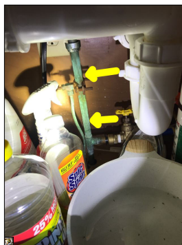
Rust/corrosion along the plumbing pipes.
