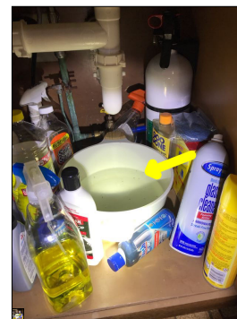
A bucket of water underneath the sink. This is considered abnormal and an indication of an active or intermittent plumbing leak.
