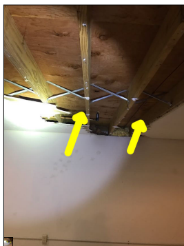
Damage along the ceiling.
