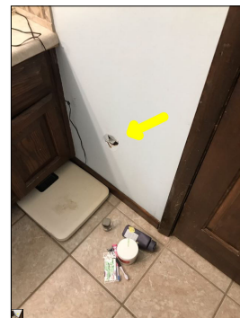
Holes/damage along the wall.
