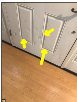
Damage/dents along the door.
