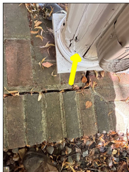
The column is loose/detached.
