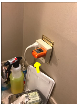
Non GFCI protected receptacles.
