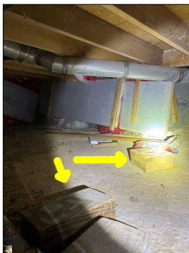
Debris and clutter within the crawl space.
