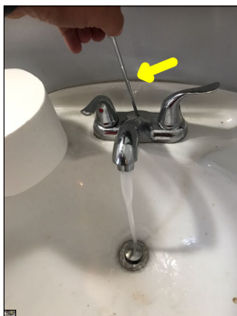
Inoperable drain stopper.
