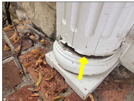
Wood rot damage along the columns. This is considered a defect. Wood rot damage is unsightly and can cause structural and property damage.
