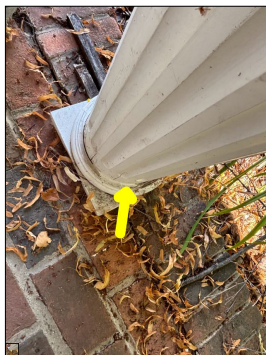
The column is loose/detached.
