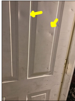
Damage/dents along the door.
