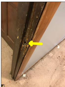
Damage along the door.
