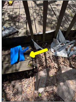
The step is loose.
