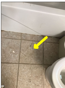
Cracked floor tiles.
