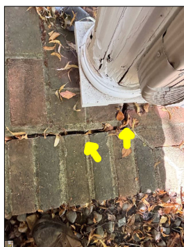
Cracks and deterioration along the porch.
