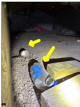
Debris and clutter within the crawl space.
