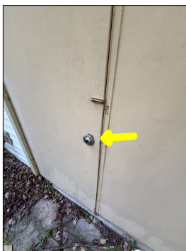
The handle is missing. Due to the missing handle, I was unable to open the door and inspect building materials behind the door.
