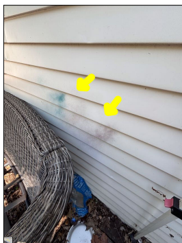
Discoloration along the siding.
