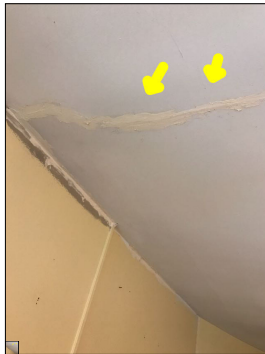
Cracks along the ceiling.
