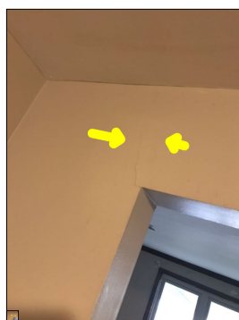
Cracks along the walls.
