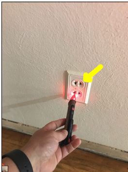
Open ground receptacles.
