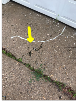
Cracks and deterioration along the driveway.
