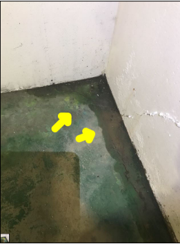
Moisture/dampness observed. This is considered a defect. An active or intermittent water source can cause mold growth and property damage.
