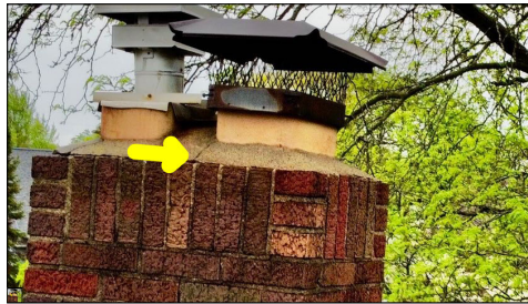
Cracks along the chimney. Cracks are considered defects and potential leak points.
