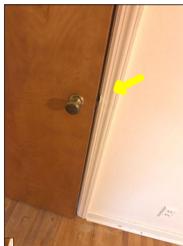
The door does not latch properly.
