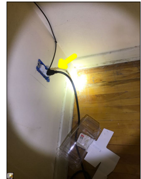
Missing receptacle cover.
