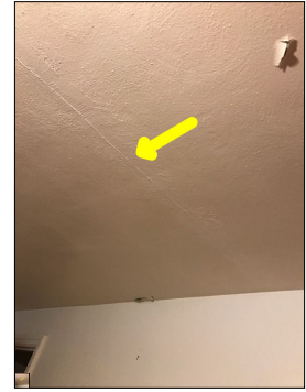
Cracks along the ceiling.
