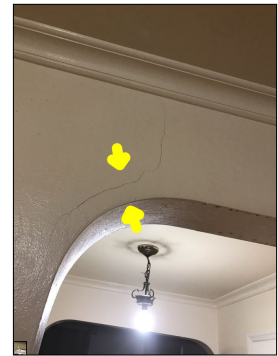
Cracks along the walls.
