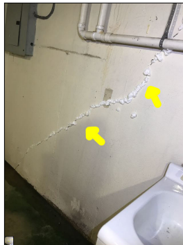
Crack along the foundation wall. Cracks are considered a defect.
