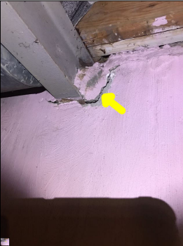
Deterioration along the foundation wall. This is considered abnormal and a defect
