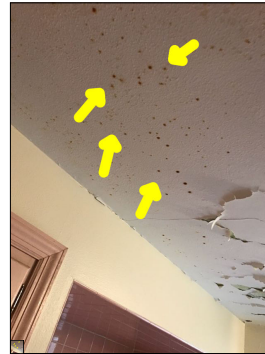
Discoloration along the ceiling. An active or intermittent water source can cause discoloration, mold growth, and property damage.
