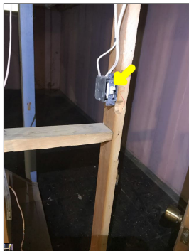
Missing switch cover.
