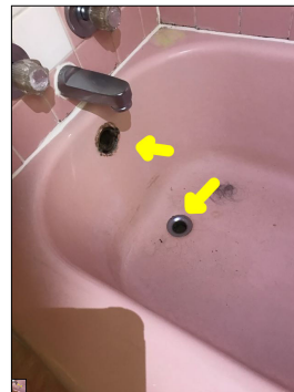
Missing drain stopper. Also, missing hardware.
