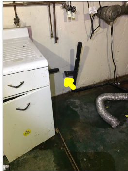
Disconnected drain pipe.
