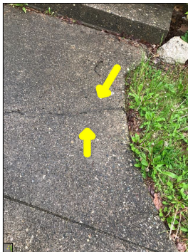
Cracks and deterioration along the service walks.
