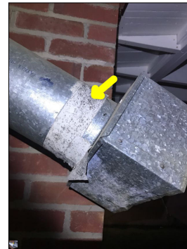
Mold like substance along the ductwork. An active or intermittent water source can cause mold growth and property damage. This is located in the basement.
