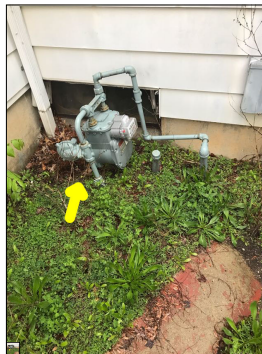
Main fuel shut off valve.
