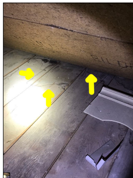
Discoloration along the sheathing. An active or intermittent water source can cause discoloration, mold growth and property damage.
