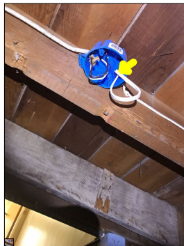
Exposed wires. This is a potential safety hazard.
