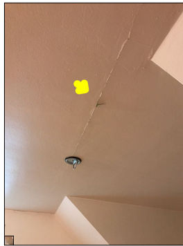
Cracks along the ceiling.
