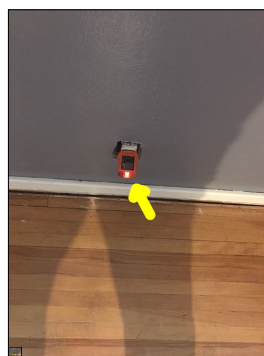
Open ground receptacles.
