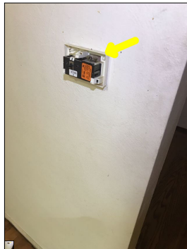
Apparent aged thermostat with missing cover.
