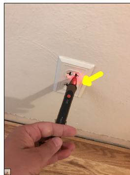
Two prong receptacles. Two prong receptacles are not grounded.
