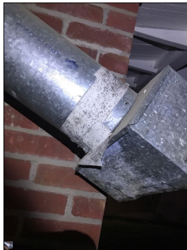
Potential asbestos based tape along the ductwork. Asbestos is a potential safety hazard.
