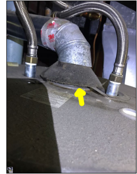
The draft hood has collapsed. This is a potential safety hazard as it can cause the water heater to not draft properly.
