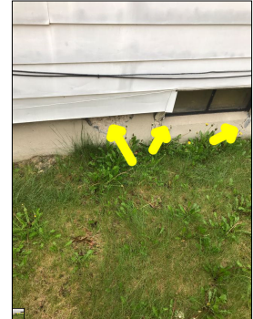
Cracks along the foundation walls. Cracks are considered a defect.
