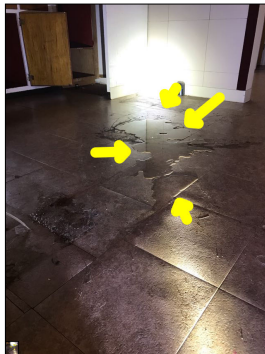
Standing water observed along the floor. This is considered abnormal and a defect. An active or intermittent water source can cause mold growth and property damage. This is an indication of a plumbing leak.
