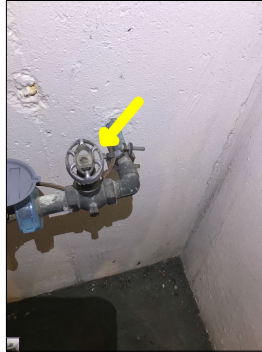
Main water shut off valve.
