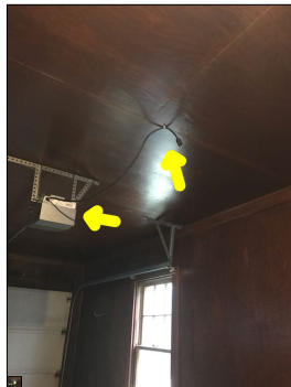
The automatic opener is inoperable. It is unplugged. It is beyond the scope of a general home inspection to plug in appliances. Doing so could potentially cause property damage.
