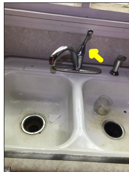
The sink is inoperable.
