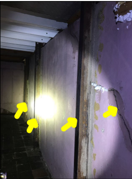
Structural modification and repairs observed along the foundation walls.
