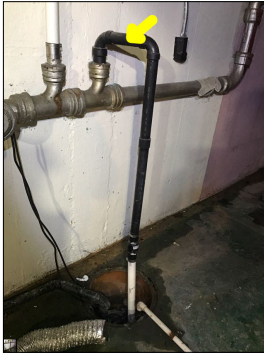
The sump pump discharges into the main drain pipes. This is not a recommended practice and does not meet the industry standard. Sump pumps should discharge to the exterior.
