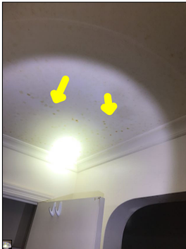
Discoloration along the ceiling. Discoloration along the ceiling is considered abnormal and a defect. An active or intermittent water source can cause discoloration, mold growth and property damage.
