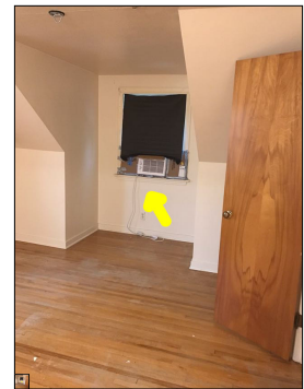
Window A/C unit observed. This is considered abnormal for a house that has central cooling. The window A/C unit is an indication that the central cooling system is unable to maintain desired interior temperatures.
