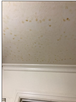
Discoloration along the ceiling. Discoloration along the ceiling is considered abnormal and a defect. An active or intermittent water source can cause discoloration, mold growth and property damage.
