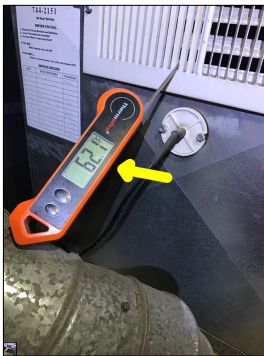
The photo identifies the temperature of the supply air while the air conditioner was in operation. The approximate temperature of the supply air was 62 degrees Fahrenheit.
