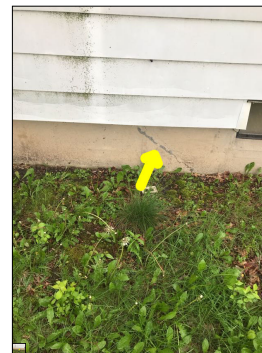
Cracks along the foundation walls. Cracks are considered a defect.
