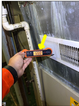
The photo identifies the temperature of the supply air while the furnace was in operation. The approximate temperature of the supply air was 122 degrees Fahrenheit.
