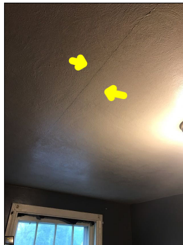
Cracks along the ceiling.
