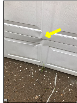
Dents/damage along the overhead garage door.
