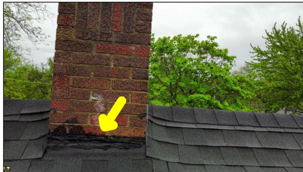
Unconventional and excessive application of roof sealant along the base of the chimney. This is considered abnormal and amateur craftsmanship. Amateur craftsmanship is prone to failure and leakage.
