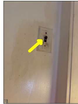
I was unable to find a function for the switch. There are no apparent lights or receptacles that are linked to the switch. This is at the top of the basement stairs.
