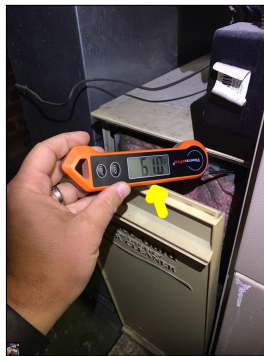
The photo identifies the temperature of the return air while the air conditioner was in operation. The approximate temperature of the return air was 61 degrees Fahrenheit.
