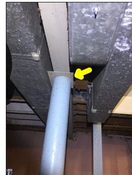
The column does not have bolts/fasteners to the beam. This is considered abnormal. Bolts/fasteners brace the column to the beam to ensure and maintain structural integrity and to prevent the column from experiencing lateral movement. The lack of proper bolts/fasteners is considered amateur craftsmanship. Amateur craftsmanship is prone to failure.
