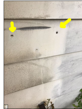
Holes along the siding.
