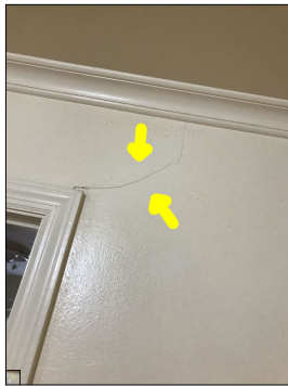
Cracks along the walls.
