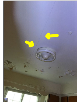
Cracks along the ceiling.
