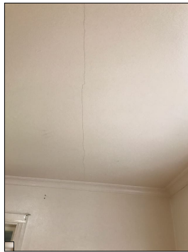
Cracks along the ceiling.
