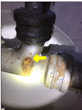
Rust and corrosion along the plumbing pipes.
