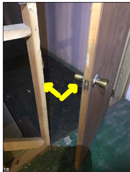
The door does not latch properly.
