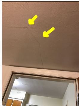
Cracks along the ceiling.
