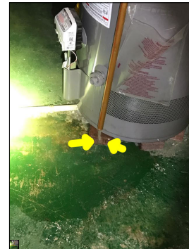
The water heater leaks. An active or intermittent water source can cause property damage and mold growth.
