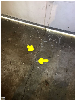
Cracks and deterioration along the floor.
