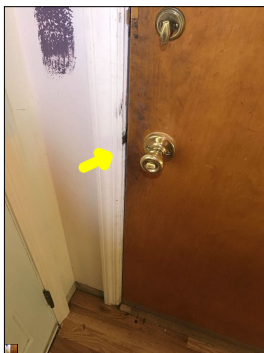
The door does not latch properly.
