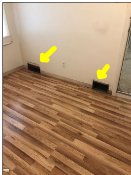
Missing vent covers.
