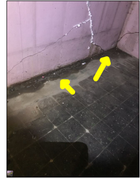
Moisture/dampness observed. This is considered a defect. An active or intermittent water source can cause mold growth and property damage.
