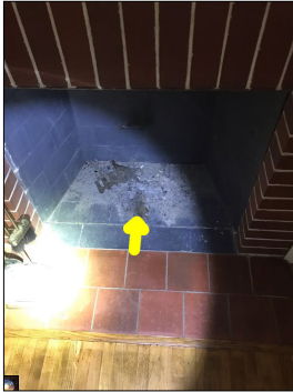
The fireplace is dirty and needs cleaning/serviced.
