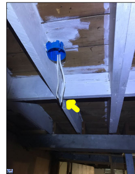
Exposed wires. This is a potential safety hazard.
