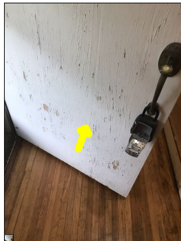
Flaking and peeling along the door.
