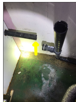
Active plumbing leak. An active or intermittent water source can cause mold growth and property damage.
