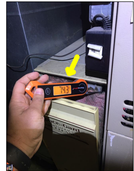
The photo identifies the temperature of the return air while the furnace was in operation. The approximate temperature of the return air was 74 degrees Fahrenheit.
