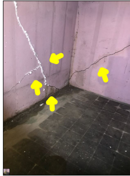
Cracks and signs of movement along the foundation walls.
