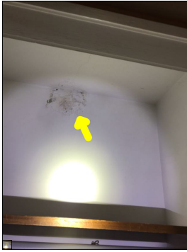
Discoloration along the ceiling and signs of previous water damage. An active or intermittent water source can cause mold growth and property damage.
