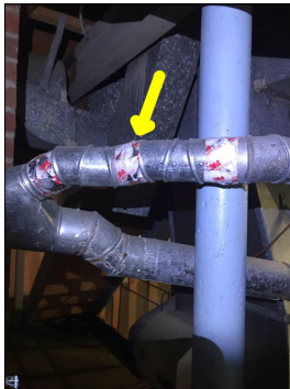
Negative sloped flue. This is not a recommended practice and is a potential safety hazard. A negative sloped flue can cause backdrafting which could cause carbon monoxide to leak into the house.
