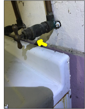
Active plumbing leak. An active or intermittent water source can cause mold growth and property damage.
