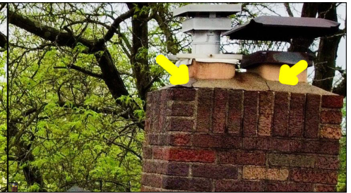
Cracks along the chimney. Cracks are considered defects and potential leak points.
