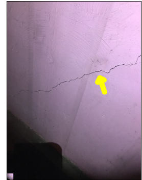
Crack along the foundation wall. Cracks are considered a defect.
