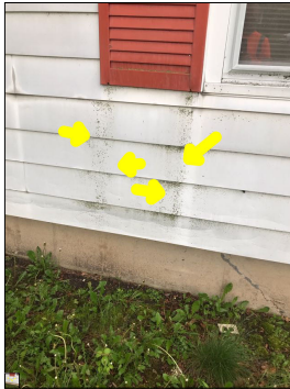
Discoloration along the siding.
