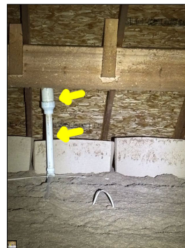
Th plumbing vent is not plumb and is crooked. This is considered abnormal and amateur craftsmanship.
