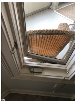
Missing window screens.
