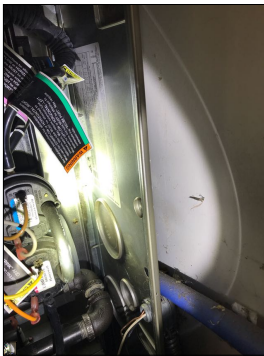
Furnace data plate.
