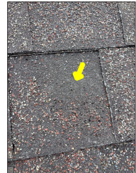
Granule loss along the roof shingles
