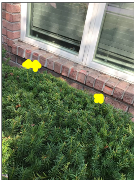
Deterioration along the brick siding.
