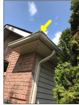
Dents/damage along the gutter system.
