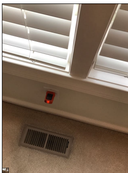
Open ground receptacles.
