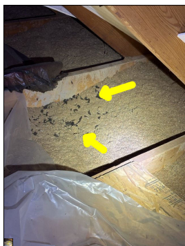
Debris and clutter within the attic. This type of debris and clutter is commonly caused by wildlife activity.
