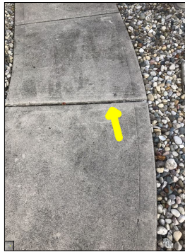
Uneven surfaces along the service walks.
