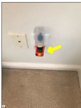
Open ground receptacles.
