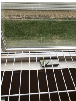
Missing window screens.
