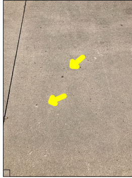
Pitting along the driveway.
