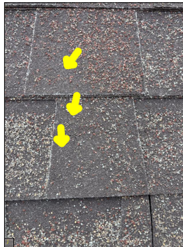
Granule loss along the roof shingles
