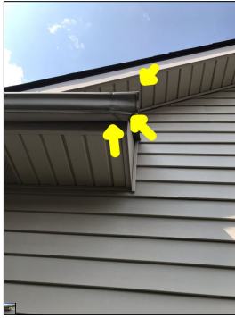
Dents/damage along the gutter system.
