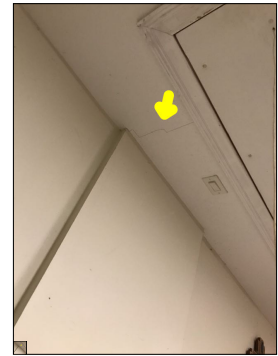
Cracks along the ceiling.
