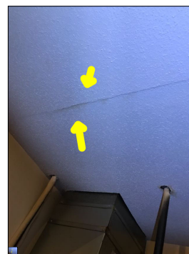
Discoloration and cracks along the ceiling.
