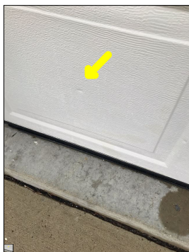
Dents/damage along the overhead garage door.
