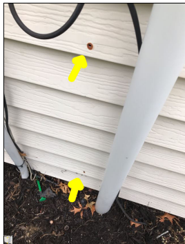
Holes along the siding.
