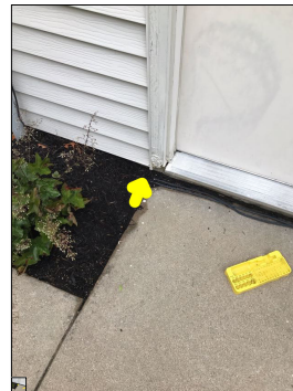
Wood rot damage.
