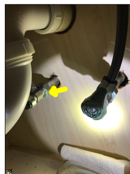
Rust/corrosion along the plumbing pipes.
