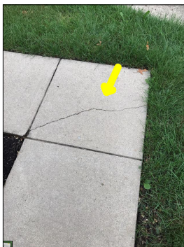
Cracks and deterioration along the service walks.
