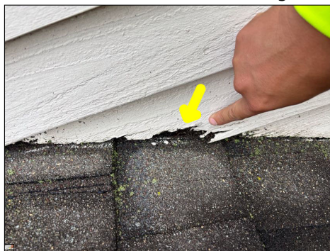
Wood rot damage.
