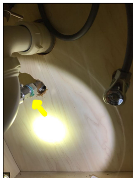
Rust/corrosion along the plumbing pipes.
