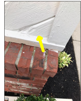
Wood rot damage.
