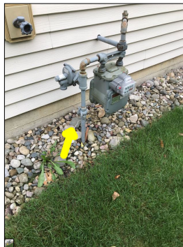
Main fuel shut off valve.
