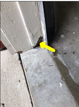
Wood rot damage.
