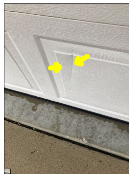
Dents/damage along the overhead garage door.
