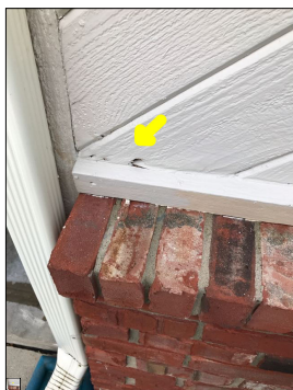
Wood rot damage.
