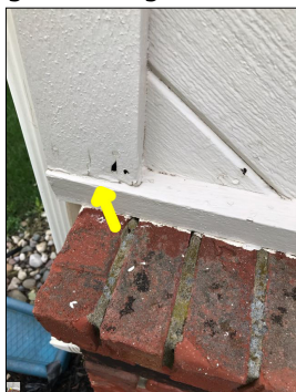
Wood rot damage.
