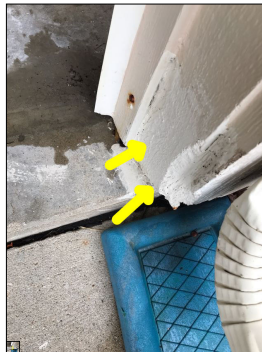
Deterioration along the siding.
