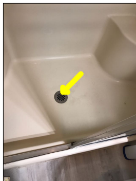
The grate is loose. This is considered a defect.
