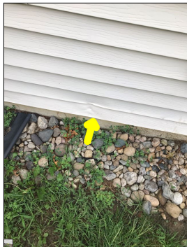
Dents along the siding.
