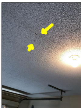
Cracks along the ceiling.
