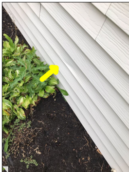
Dents along the siding.
