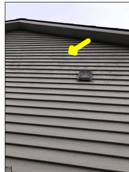
Discoloration along the siding.
