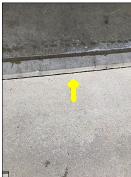
Uneven surfaces along the driveway.
