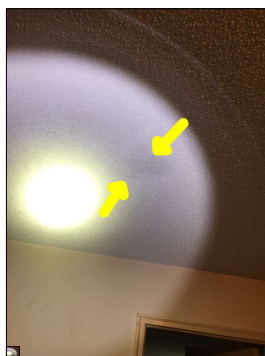
Areas along the popcorn ceiling are falling off.
