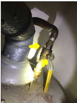
Corrosion along the water supply lines.
