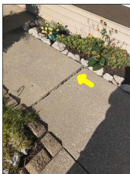
Uneven surfaces along the service walks.
