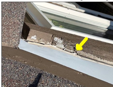
Gaps along the siding.
