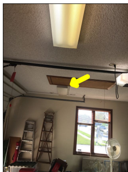
The light is inoperable.
