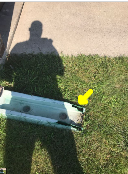
Damaged splash block.
