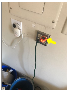
Non GFCI protected receptacles.
