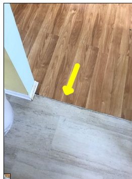
Missing trim pieces along the floor.
