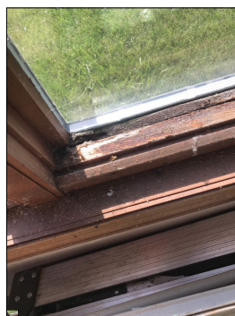
Wood rot damage along the window.
