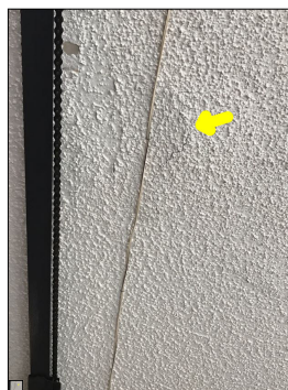
Cracks along the ceiling.
