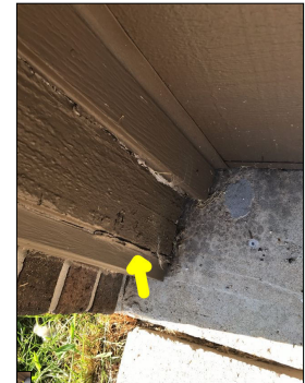
Gaps along the siding.
