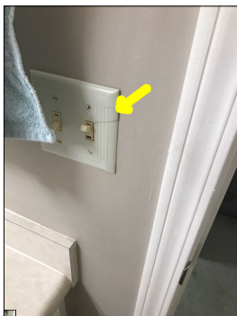
Cracked switch cover.
