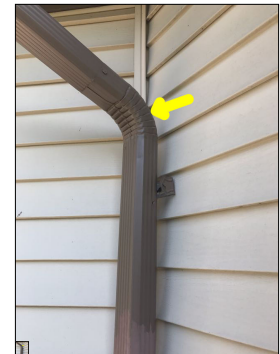
The downspout is loose.
