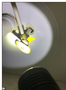
Rust/corrosion along the plumbing pipes.
