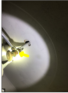
Rust/corrosion along the plumbing pipes.
