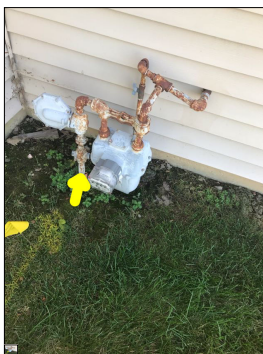
Main fuel shut off valve.
