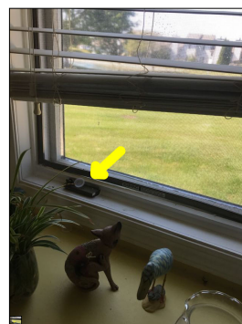
Detached window crank. The window is inoperable.
