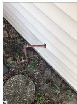
Holes along the siding.
