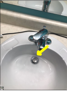
Inoperable drain stopper.
