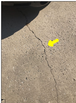
Cracks and deterioration along the driveway.
