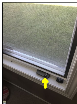
Detached window crank. The window is inoperable.
