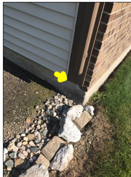
Missing downspout elbows.
