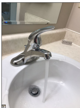
The faucet is loose.
