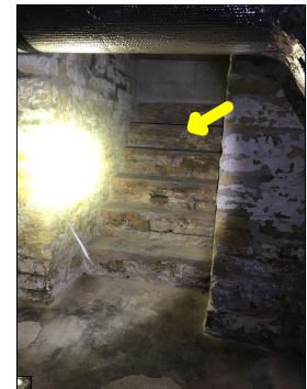
Old stair case observed.
