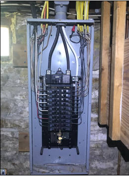
General photo of the circuit breaker panel.
