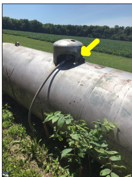
Main fuel shut off valve.
