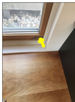
Discoloration along the window. An active or intermittent water source can cause discoloration, mold, and property damage.
