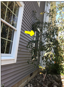
Vegetation against the siding/in proximity of the siding. This is not a recommended practice. Vegetation has the potential to harbor insects, wood destroying insects, rodents and hold moisture. Insects, wood destroying insects, rodents and moisture have the potential to create future problems for a house, such as structural damage, pest infestation and wood rot damage.
