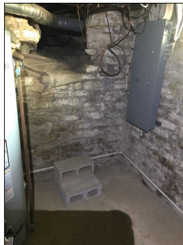
Field stone foundation observed in some areas. Field stone foundations no longer meet modern day structural standards. Field stone foundations are considered aged. Potential repairs to stone foundations and water intrusion from field stone foundations should not be a surprise.
