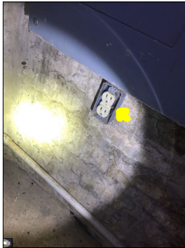
Missing receptacle cover.
