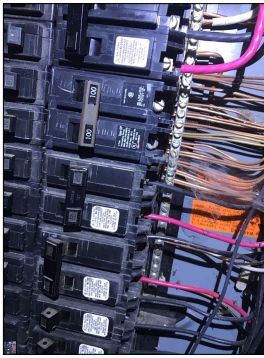
Unused circuit breaker.
