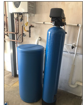
Water softener within the detached garage/pole barn.
