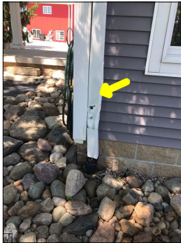
Dents/damage along the gutter system.
