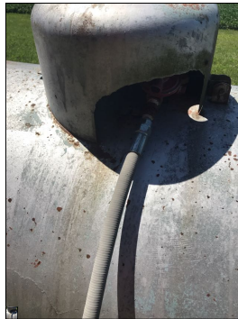
Rust and corrosion along the fuel tank. Rust and corrosion can create holes along the tank, thus creating a fuel leak.
