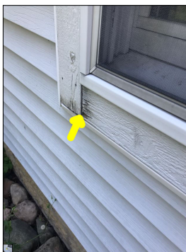
Wood rot damage.
