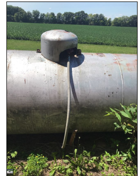
Gas smell noticed when inspecting the tank. This is a potential safety hazard.
