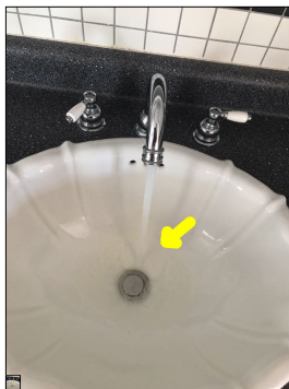
Inoperable drain stopper.
