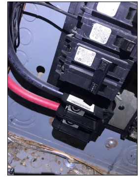
Unused circuit breaker.
