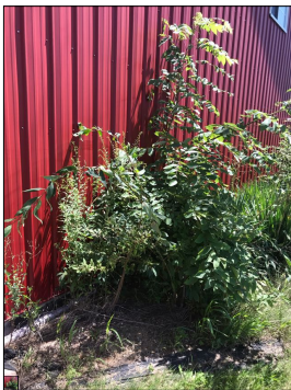
Vegetation against the siding/in proximity of the siding. This is not a recommended practice. Vegetation has the potential to harbor insects, wood destroying insects, rodents and hold moisture. Insects, wood destroying insects, rodents and moisture have the potential to create future problems for a house/structure such as structural damage, pest infestation and wood rot damage.
