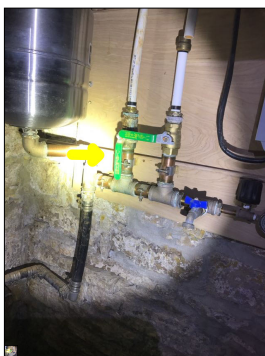
Apparent main water shut-off valve.
