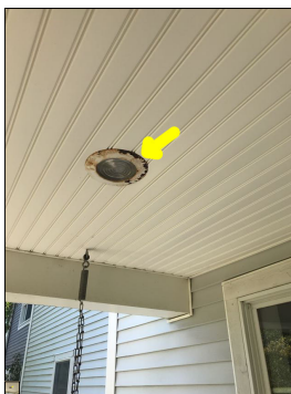
Rust and corrosion along the exterior lights.
