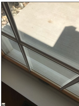
Missing window screens.
