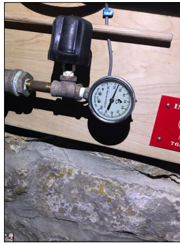
The well pressure was approximately 25 PSI during the inspection.
