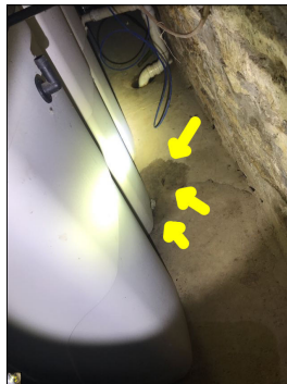
Moisture/dampness observed under the water softener. An active or intermittent water source can cause damage, mold, water damage. No active leaks in this area observed on the day of the inspection. Recommend licensed plumber further evaluate and make necessary repairs.
