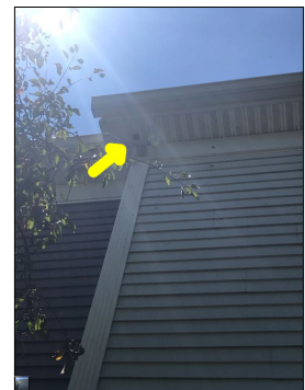
Hole along the siding.
