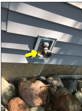
Discoloration along the siding.
