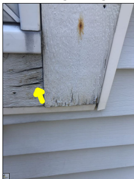
Wood rot damage.
