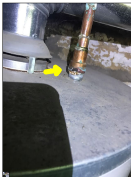
Corrosion along the water supply lines.
