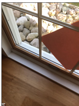
Missing window screens.
