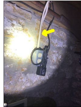
The wires along the concrete/stone are not wrapped in conduit. This is considered abnormal, amateur craftsmanship and a potential safety hazard. The wires can absorb moisture from the concrete/stone, thus causing arcing, spark and/or fire.
