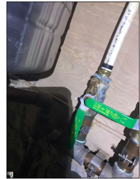
Rust and corrosion along the water supply lines. Also, moisture observed in the area. This is considered an active plumbing leak. An active or intermittent water source can cause mold growth and property damage.
