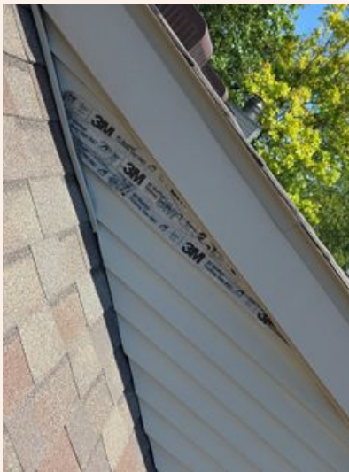
Damage or missing piece of siding that has been covered up with tape on the upper west side of the rear Dormer
