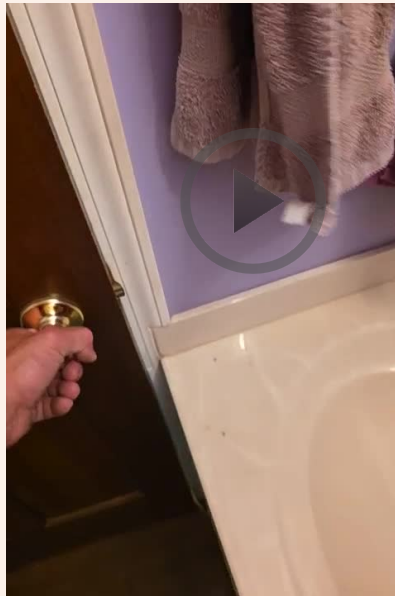
(This video is only viewable online.) Main floor hallway bathroom door does not close
