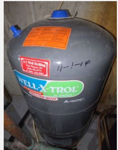
Pressure tank for the well system
