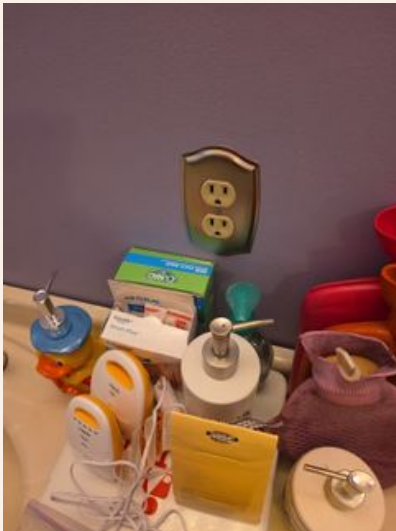
Main floor hallway bathroom outlet is not GFCI protected
