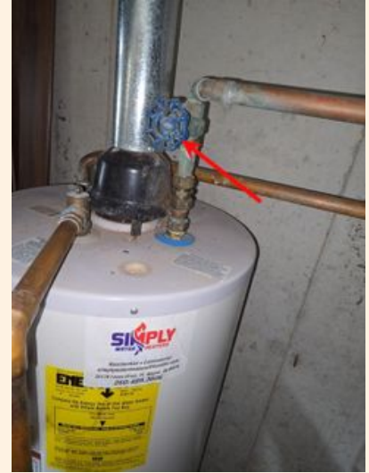
Cold water supply shut off to the water heater
