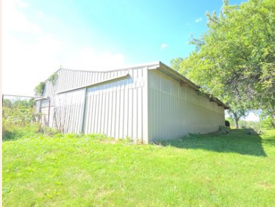
Barn is missing gutters and downspouts on both sides
