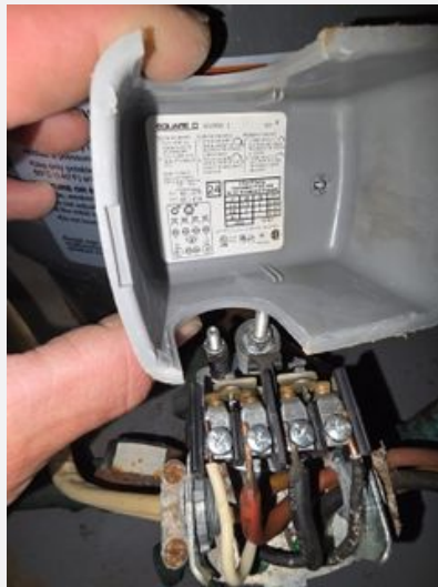
Pressure switch nameplate
