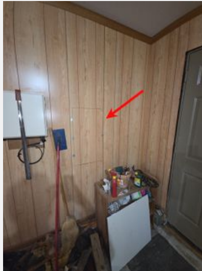
Main Electric panel is hidden behind paneling door in the southwest corner of the attached garage
