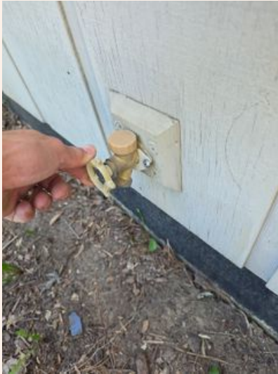
Exterior water spigot on the front of the house was not working at the time of the inspection
