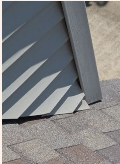
Vinyl siding has come untucked from the outside vinyl corner post on the Lower West rear Dormer
