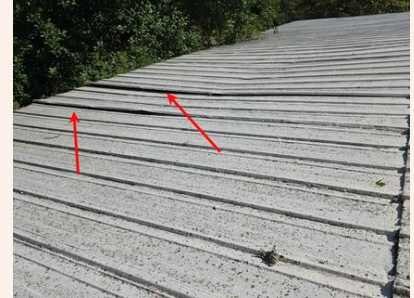
Metal roofing panels that have come loose on the east ends of the barn roof
