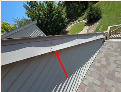
Fascia flashing on the Second Story West rake towards the back is overlapping the wrong way
