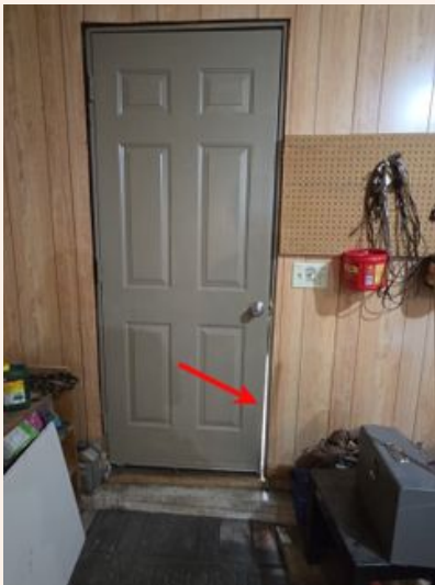
Light can be seen through the bottom right of the garage door
