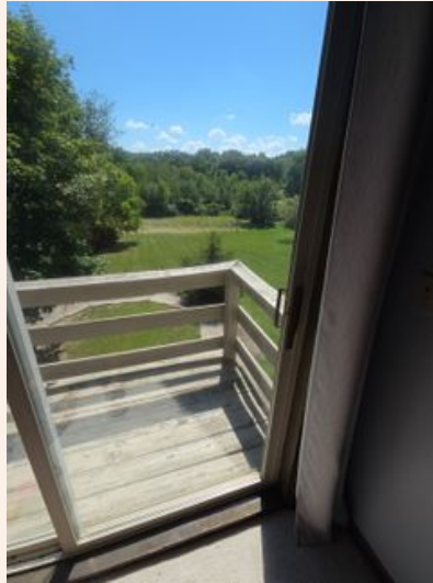
Second floor balcony sliding patio door does not lock
