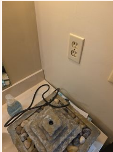
Half bathroom basement Outlet not GFCI protected
