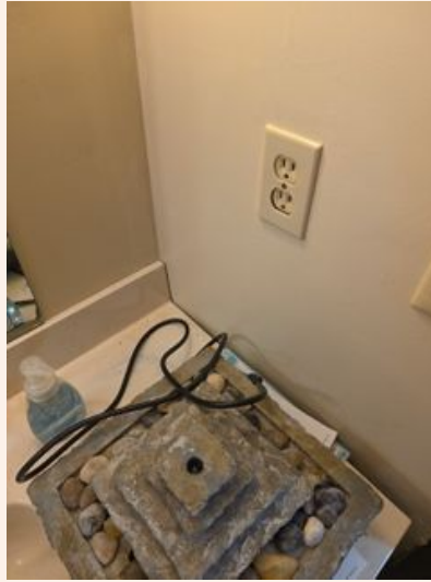
Half bathroom basement Outlet not GFCI protected
