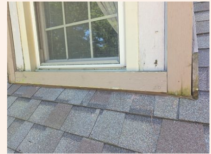
Wood trim board around the front North facing Dormers as well as the Dormers fascia board are in need of maintenance and sealing
