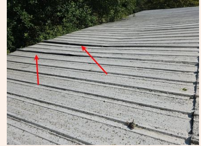
Metal roofing panels that have come loose on the east ends of the barn roof
