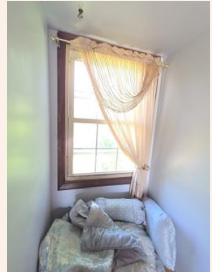
Was unable to open the front facing north window in the East Dormer
