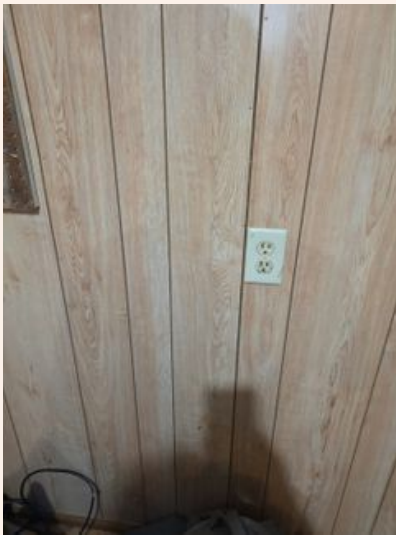
Attached garage Outlets are not GFCI protected
