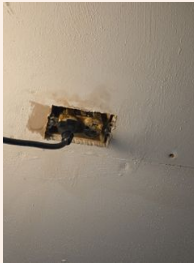
Outlet for the garage door opener in the attached garage is missing a cover
