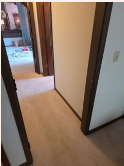
Second floor West bedroom is missing a door
