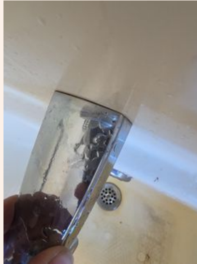
Second floor bathroom tub spout needs sealant between it and the wall or a small Gap can be seen
