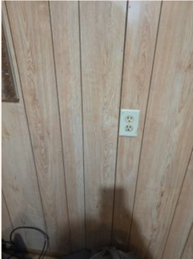
Attached garage Outlets are not GFCI protected
