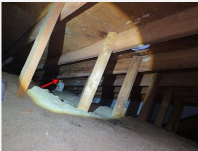
PVC plumbing vent
