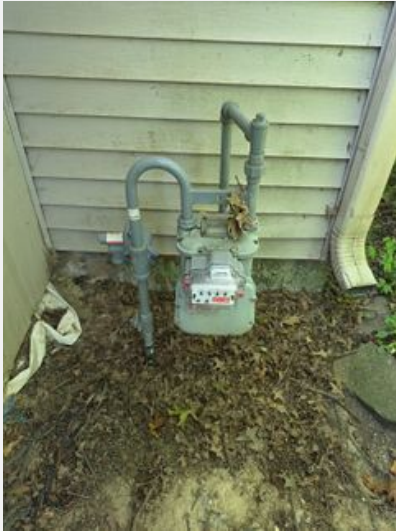
Gas meter and Main gas supply shut off to the property located on the exterior front northeast corner of the house
