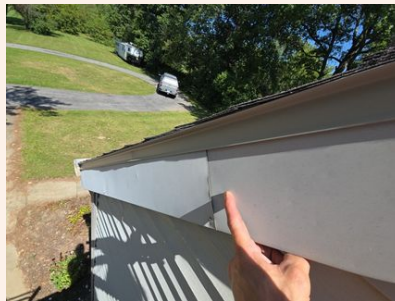
Fascia flashing on the Second Story West rake towards the front is overlapping the wrong way
