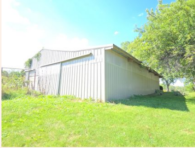
Barn is missing gutters and downspouts on both sides
