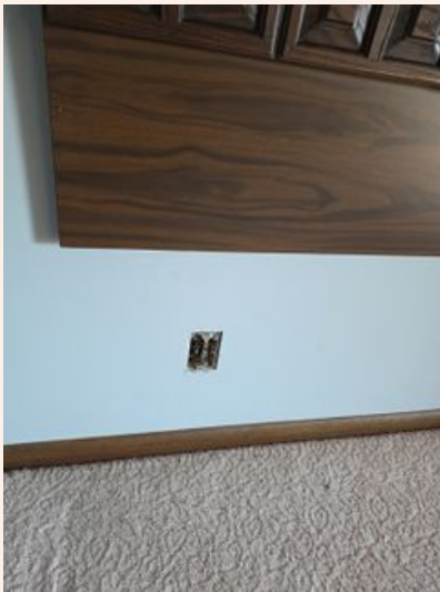
Damaged Outlet and missing cover in the second floor east bedroom on the East wall
